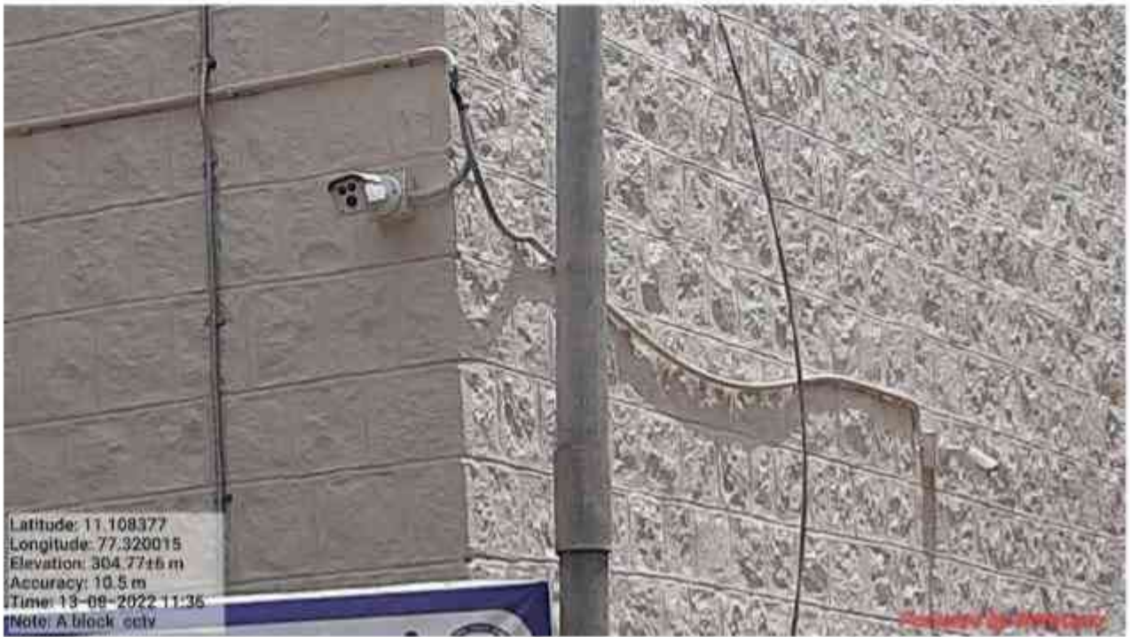
CCTV IN A BLOCK
