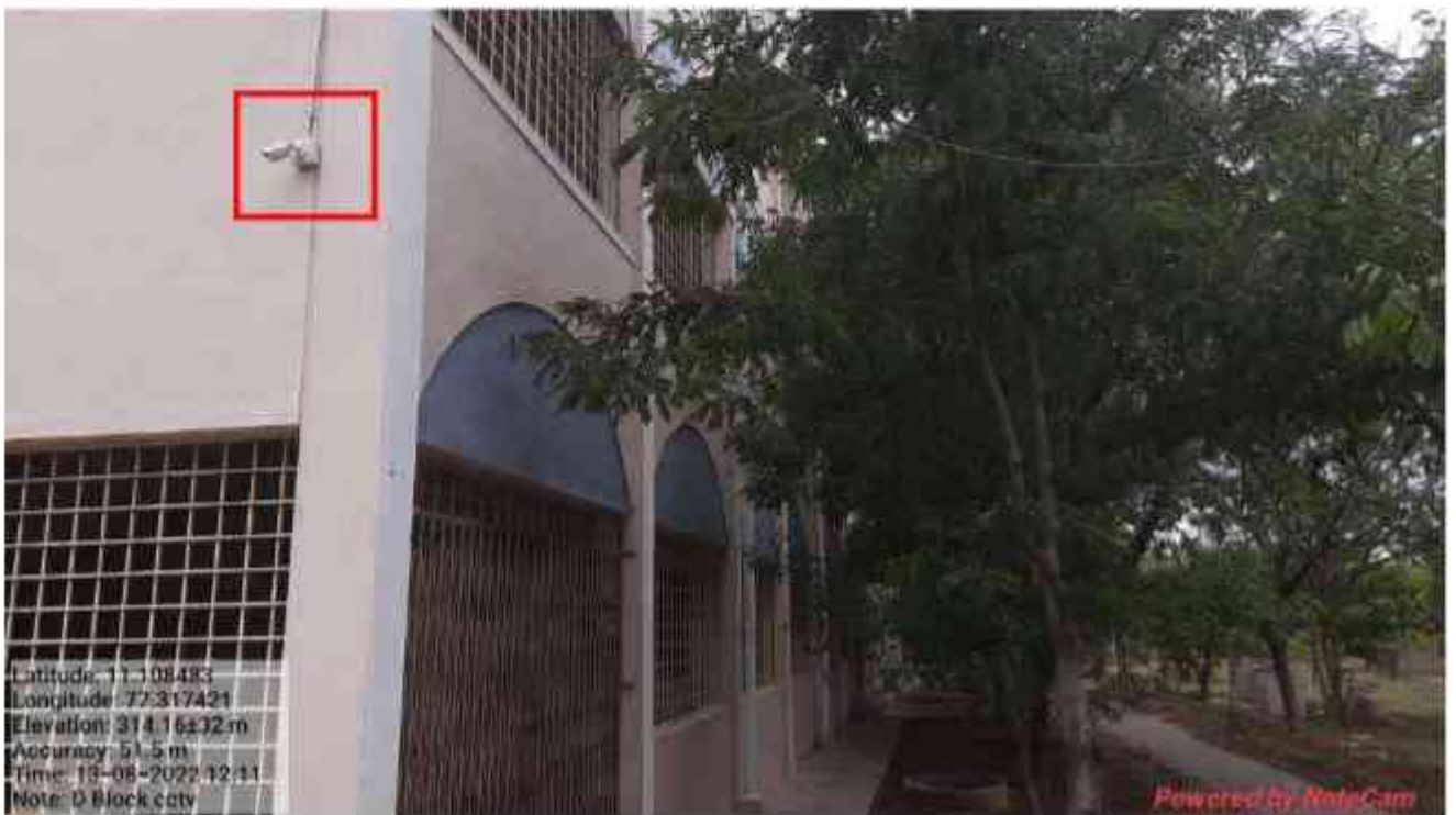
CCTV IN D BLOCK
