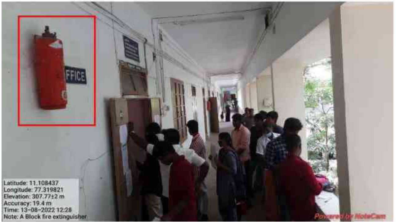
FIRE EXTINGUISHER IN A BLOCK
